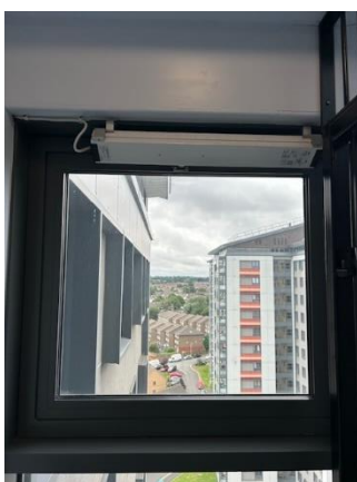
AOV window in stairs lobby
