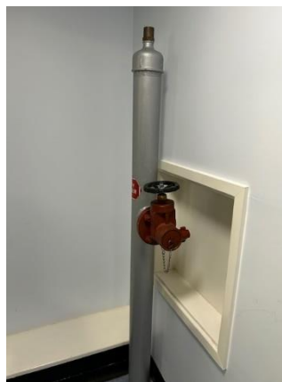
Dry riser outlets all levels
