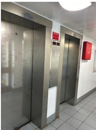
x2 passenger lifts
