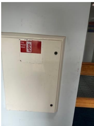
Dry riser inlet
