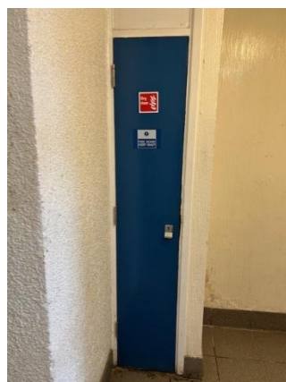
Dry riser inlet cupboard
