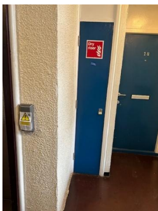
Dry riser outlet cupboard
