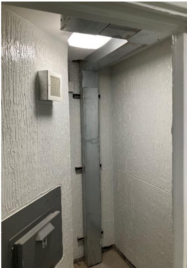
Figure 28: Refuse room - hopper and extract
