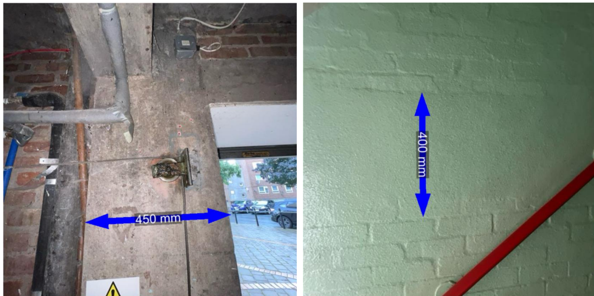
Figure 13 and 14: Vertical and Horizontal RC Structure Visible
