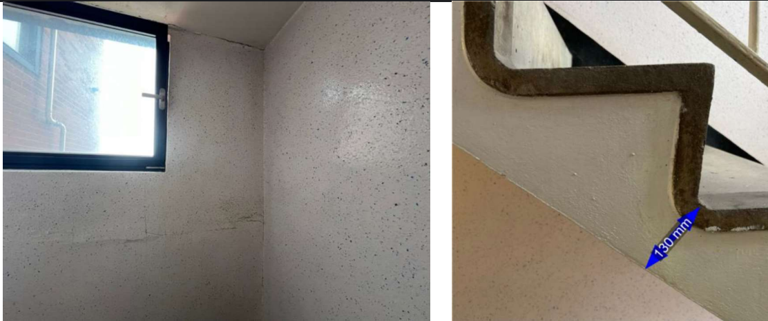
Figure 13 and 14: BRE 1 crack within stair core and staircase
