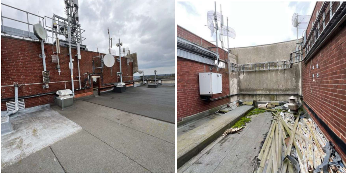
Figure 11 and 12: Roof level enclosure and debris
