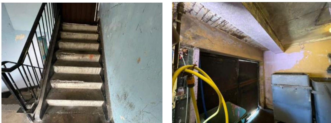
Figure 15 and 16: Defects to RC Structure
