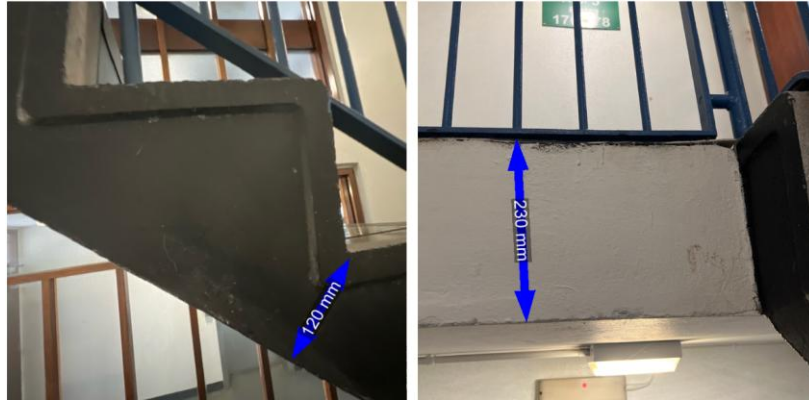
Figure 14 and 15: Slab edge and stair stringer
