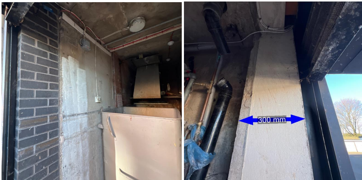
Figure 15 and 16: RC soffit and vertical column
