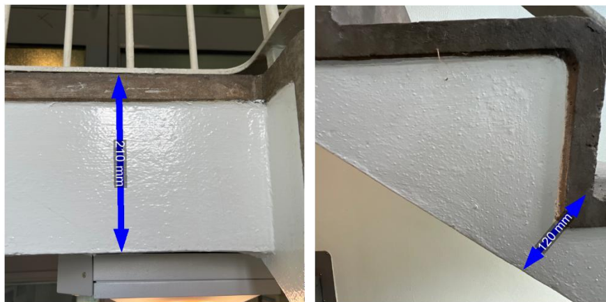
Figure 14 and 15: Stair stringer and concrete slab
