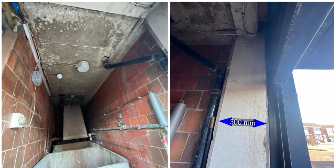
Figure 15 and 16: RC soffit and vertical column
