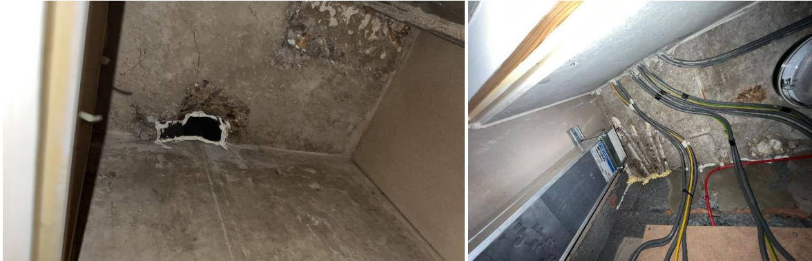
Figure 13 and 14: Localised areas of spalling
