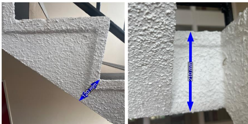
Figure 14 and 15: Stair Stringer and Landing
