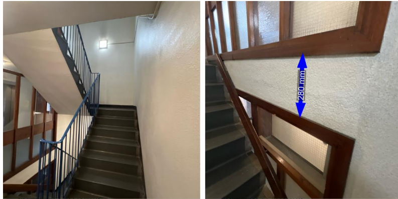
Figure 14 and 15: Slab edge and stair stringer
