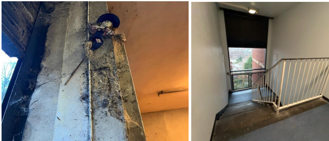
Figure 14 and 15: Localised area of spalling and Staircase
