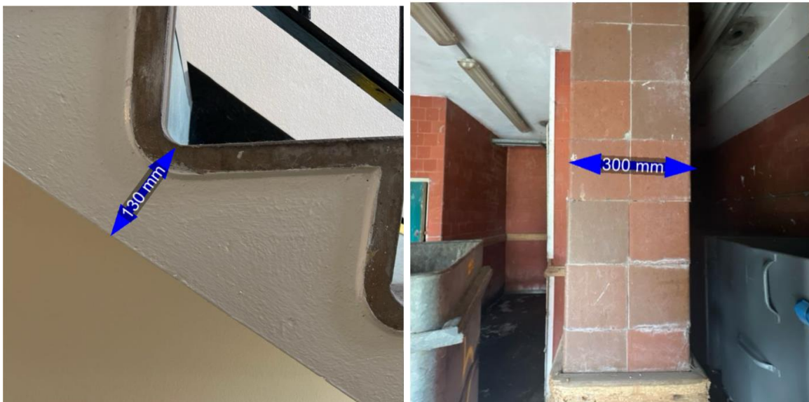
Figure 15 and 16: Staircase Stringer and clad column at ground floor
