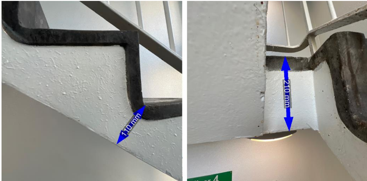
Figure 13 and 14: Stair stringer and concrete slab
