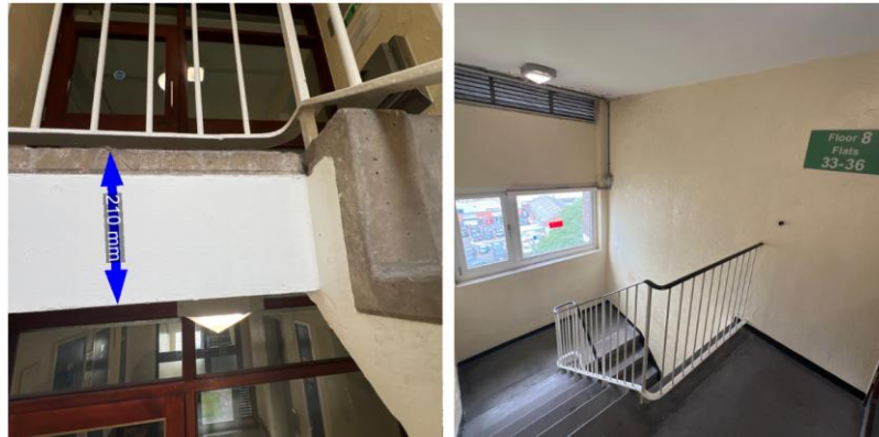
Figure 14 and 15: Slab edge and stair stringer
