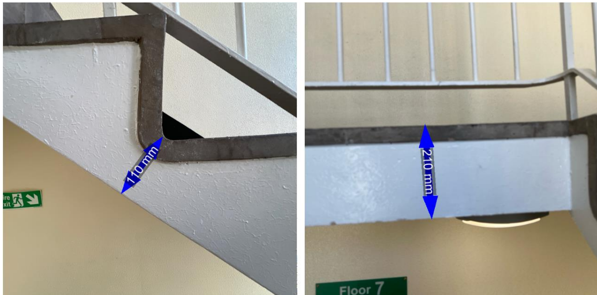
Figure 13 and 14: Stair stringer and concrete slab
