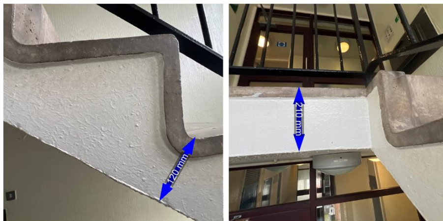
Figure 14 and 15: Slab edge and stair stringer
