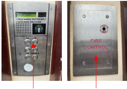
Intercom access and firefighter's switch
