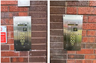
Both entrance door access systems.
