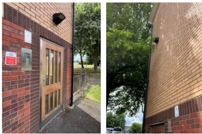
Lighting units above entrances to the block.
