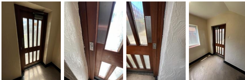
Final front exit doors and doors exits buttons
