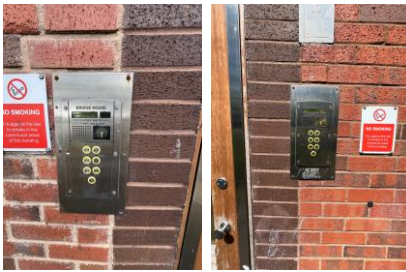
Both entrance door access systems.
