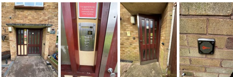
Front and rear entrance doors with access system.
