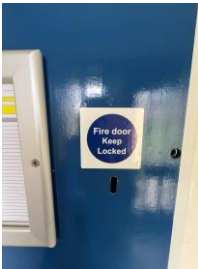
Fire signage on electrical cupboard
