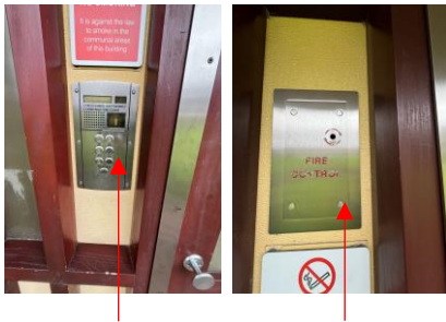
Intercom access and firefighter's switch
