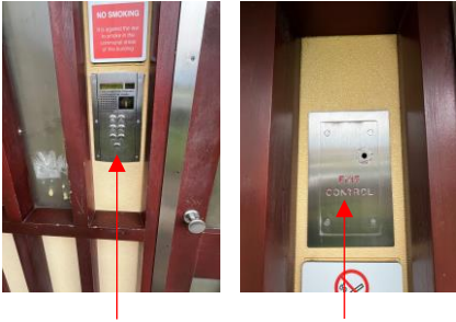
Intercom access and firefighter's switch
