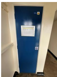
Fire signage on electrical cupboard
