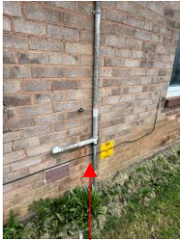
External Gas supply
