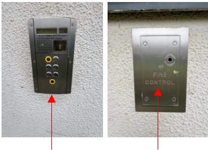
Intercom access and firefighter's switch
