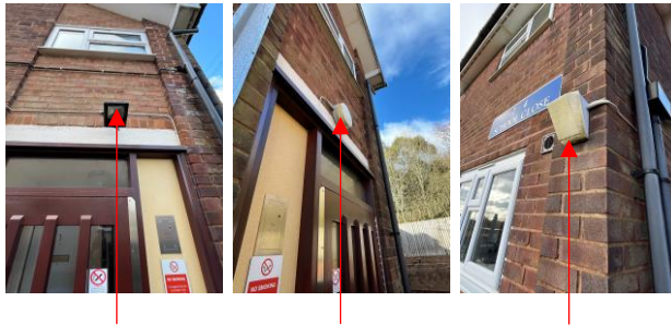
Front external lighting to flats 1-3 and 2-4
