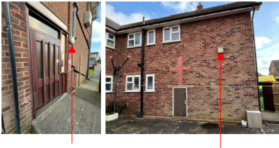
Front and rear external lighting
