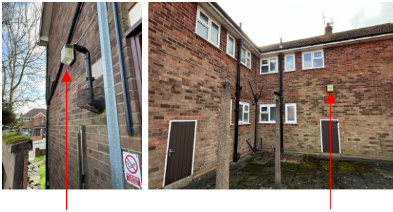
Front and rear external lighting
