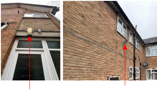
Front and rear external lighting.
