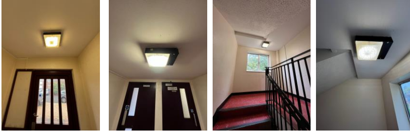
Communal area, stairwell emergency lighting
