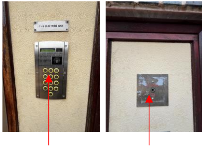
Intercom access and fire-fighter's switch
