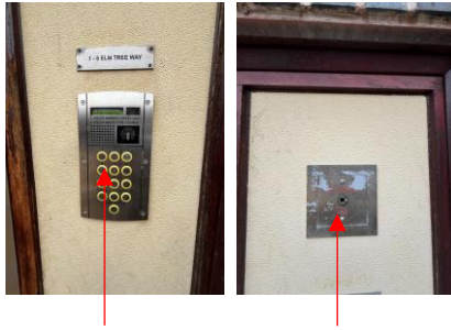
Intercom access and firefighter's switch
