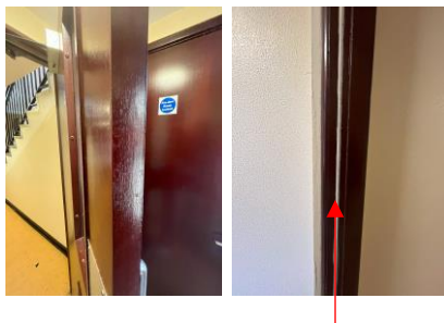
Fd30s and intumescent strip
