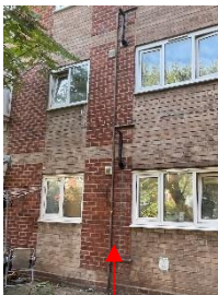
External Gas supply
