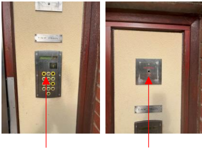
Intercom access and firefighter's switch
