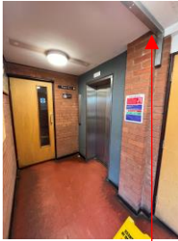
Metal Electrical Trunking
