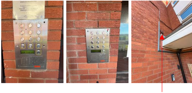
Intercom access and firefighter's lift override switch.
