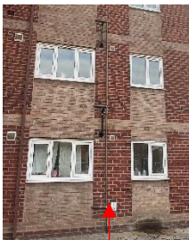
External Gas supply
