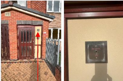
Firefighters override switch
