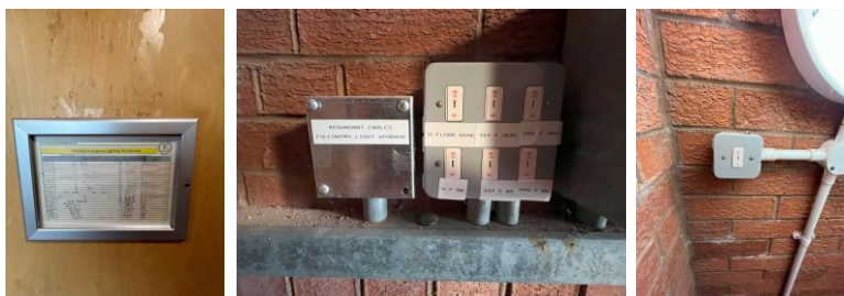
Monthly Sandwell test record and testing switches
