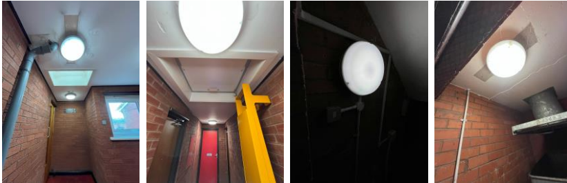
Communal area, service and refuse cupboard emergency lighting
