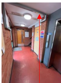
Metal Electrical Trunking
