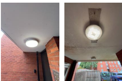
Front External lighting
