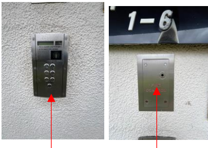
Intercom access and firefighter's switch
