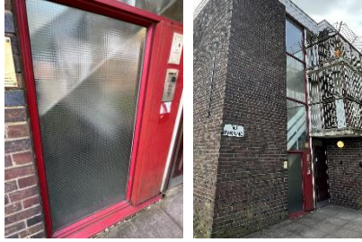
Georgian wired glass to stairwells
