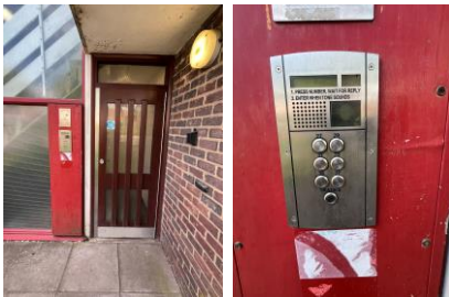
Front entrance door with access system.
