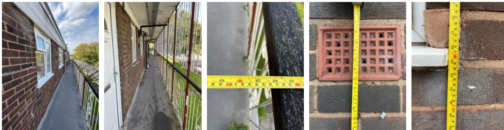
1 st and 2 nd floor open deck with width and height of air brick and windows
