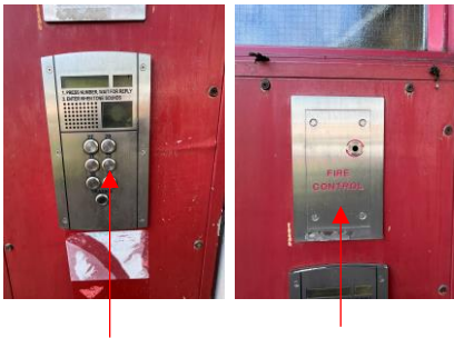
Intercom access and firefighter's switch
