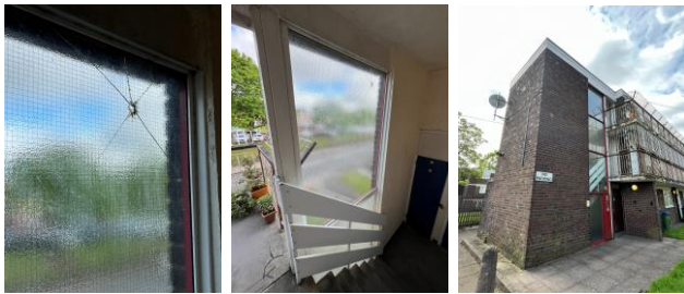
Damaged section of glazing on the 2 nd floor.
