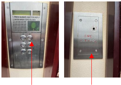
Intercom access and firefighter's switch
