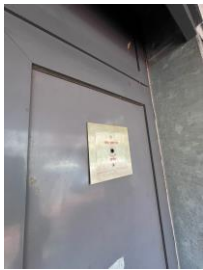
Firefighter's switch is only present at the front entrance
