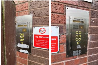
Both entrance door access systems.
