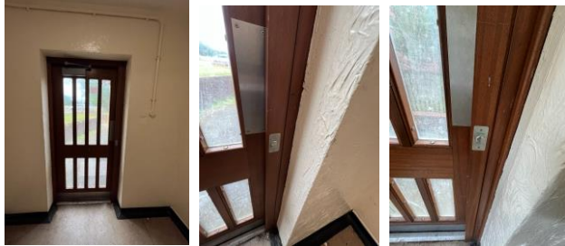
Final front exit doors and doors exits buttons
