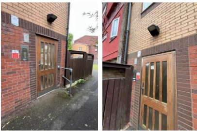
Lighting units above entrances to the block.
