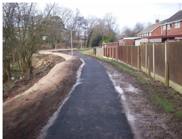
Figure 3 - Defence bund and wall installed adjacent to the River Stour at Grange Crescent, Halesowen in 2012, in partnership with the Environment Agency
