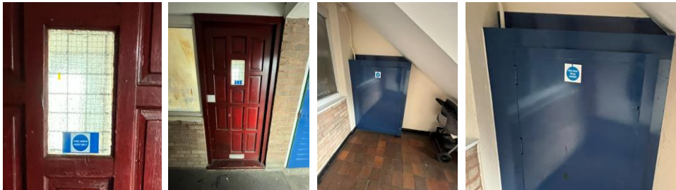
Fire signage on electrical cupboard
