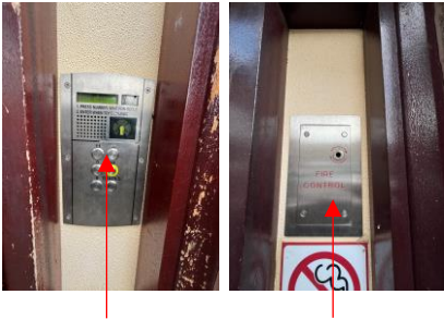
Intercom access and firefighter's switch
