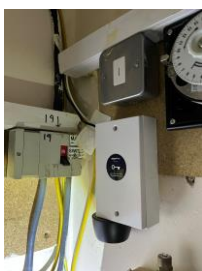
Emergency light test switch
