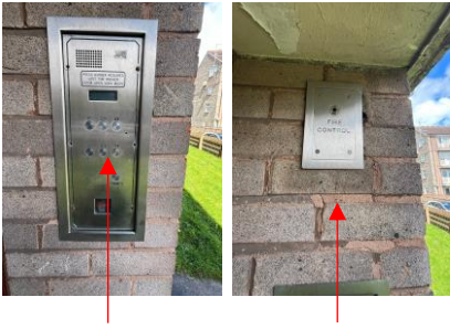
Intercom access and firefighter's switch
