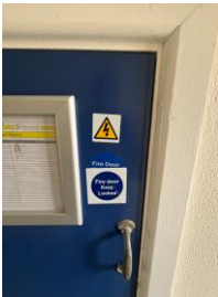
Fire signage on electrical cupboard
