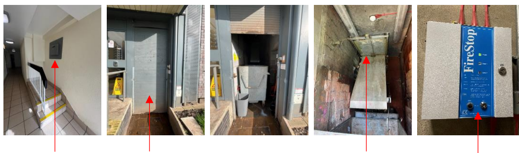
Bin chute, access via shutter, refuse chute closure plate and suppression system
