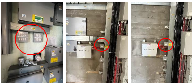
Ground, 2 nd and 5 th floor emergency light test switches
