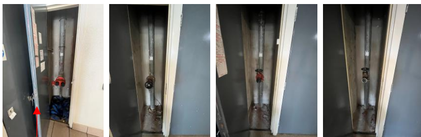
FD30s door and example of riser valves from floors, G,1,2,3,
