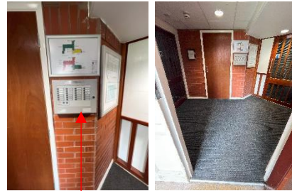
Repeater Fire alarm panel
