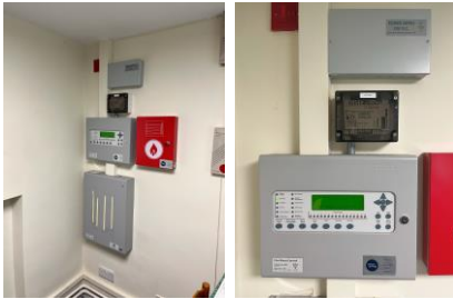
Main fire alarm panel
