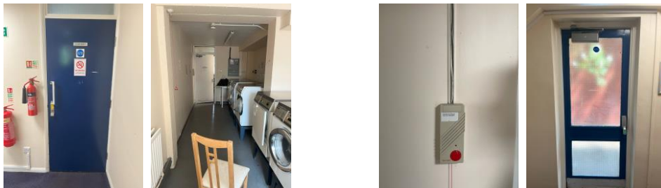
Community alarm link & fire exit
